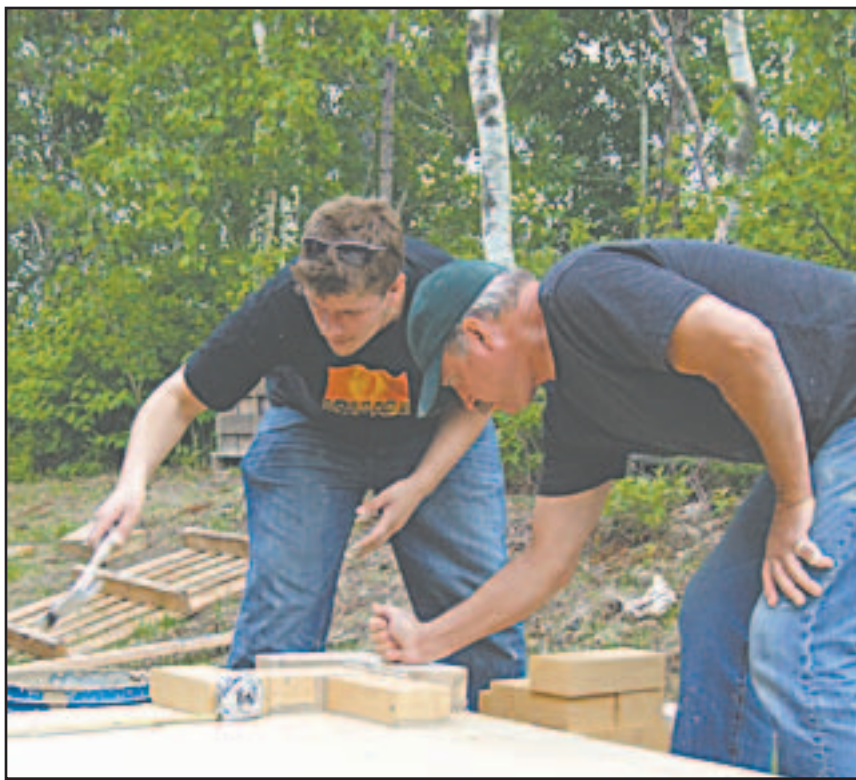
Anna Kurth Jered Dodson and Don Hedman work on building a soda kiln last week at Hibbing Community College.
